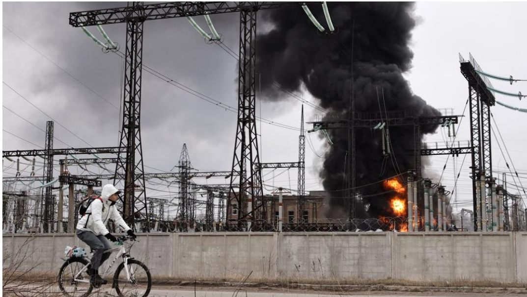
A man rides a bicycle past an energy infrastructure facility attacked by Russia in Kharkiv, Ukraine, March 22, 2024. AP/Yevhen Ti
